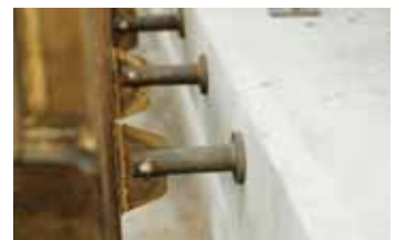
Above: Installation of the screen; metal rods attach the screen to the building. Main photo: Close up of bronze screen showing the cast glass detail.
