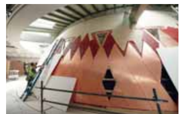
Above: The courtroom's steel framework; wooden panels during installation in the interior; installation of the copper panels on the courtroom exterior. Main photo: Courtroom interior showing the detail of the panelling.
