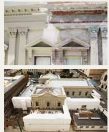
Above: Plastering before and after, the building surrounded with the polystyrene screen. Main photo: The Old High Court Building's main entrance on Stout Street.
