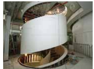
Above: Progress photos show the staircase's steel structure. Main photo: Completed staircase.
